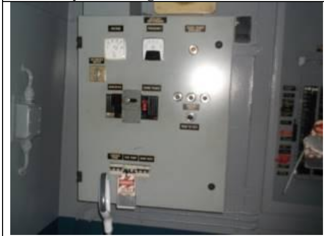
13 Main Switch Gear
