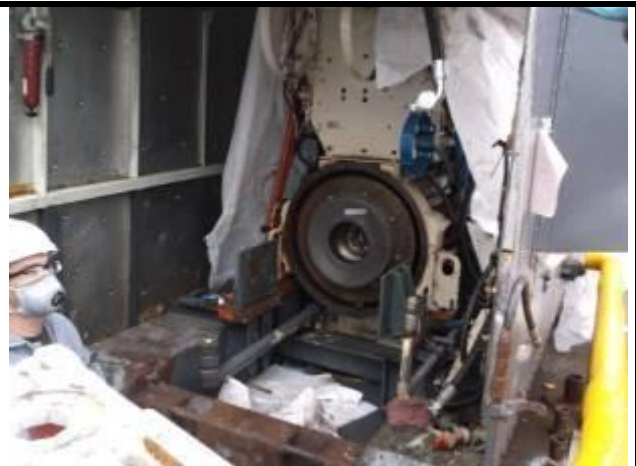
04 Typical Propulsion Engine
