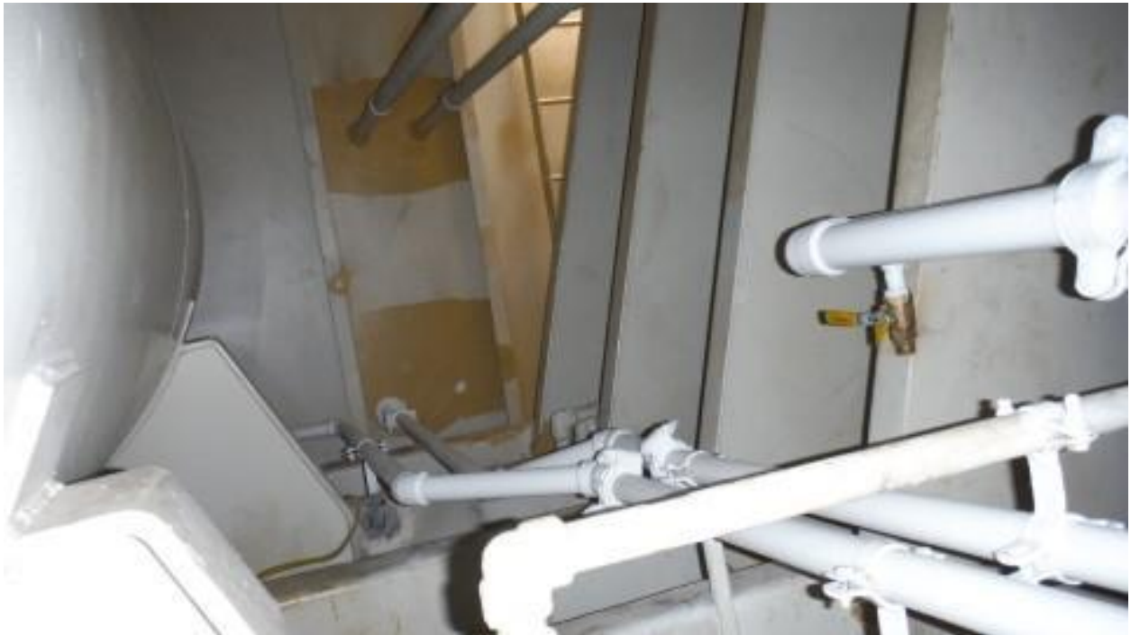
Fuel Oil Tanks Void # 3
