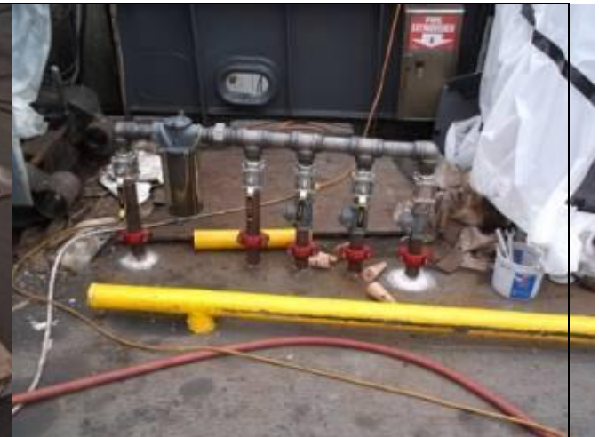
06 New Bilge Washdown Manifold
