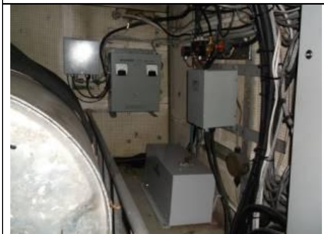
15 Potable Water Tank & Battery Charger
